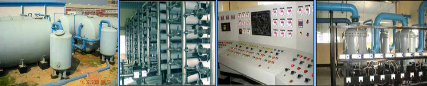
400 M 3 /hour Combined Plant with 320 M 3 /hour Reverse Osmosis Plant Karnaphuli SEZ, Chittagong
