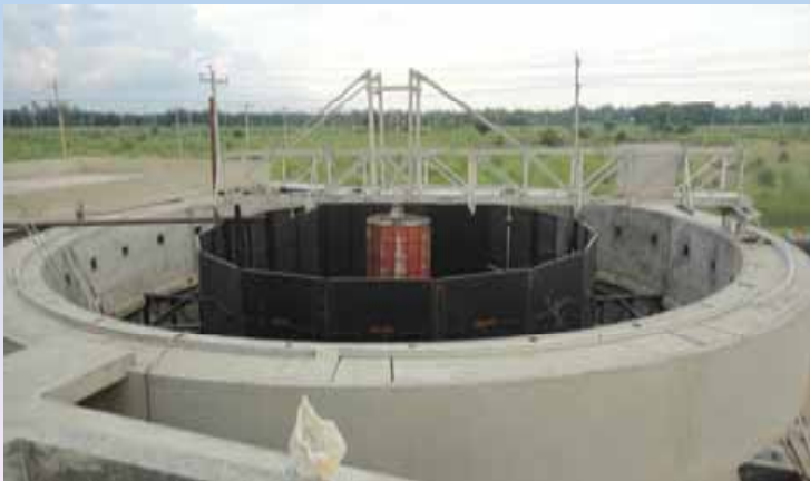
5 MGD (950 M 3 /hour Water Treatment Plant BSCIC Tannery Project, Savar
